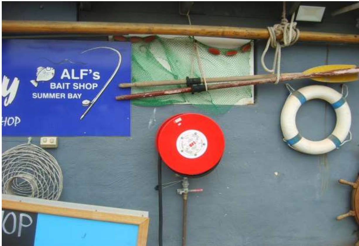
Photo 8 – Indicates a First-Aid Fire Hose Reel located outside Barrenjoey Boat Hire on the Northern façade of the existing structure (Steve Brooks 2020)
