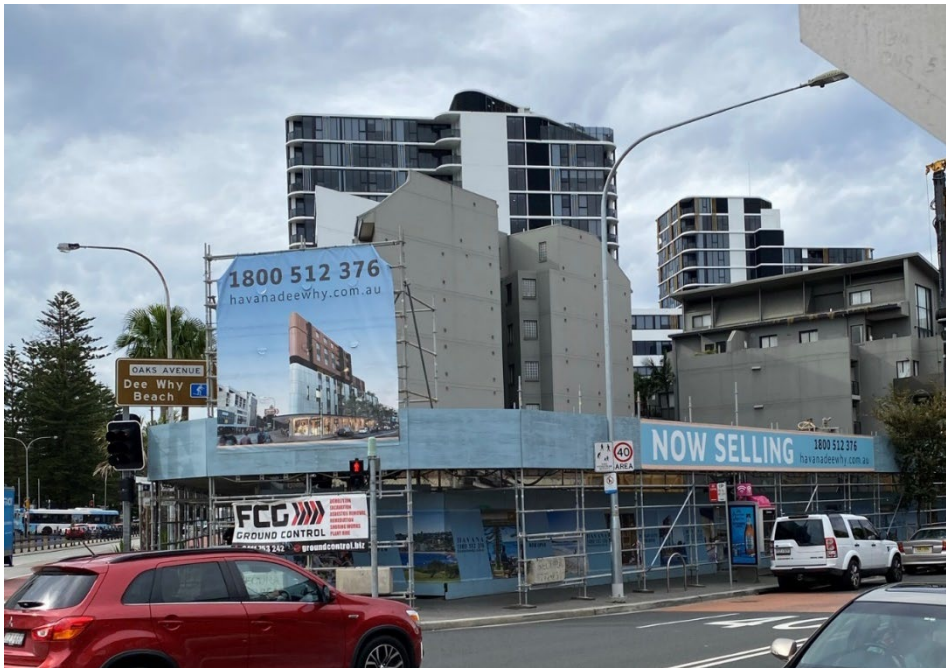
Photograph 4: Corner of Pittwater Road and Oaks Avenue, where site redevelopment has commenced
