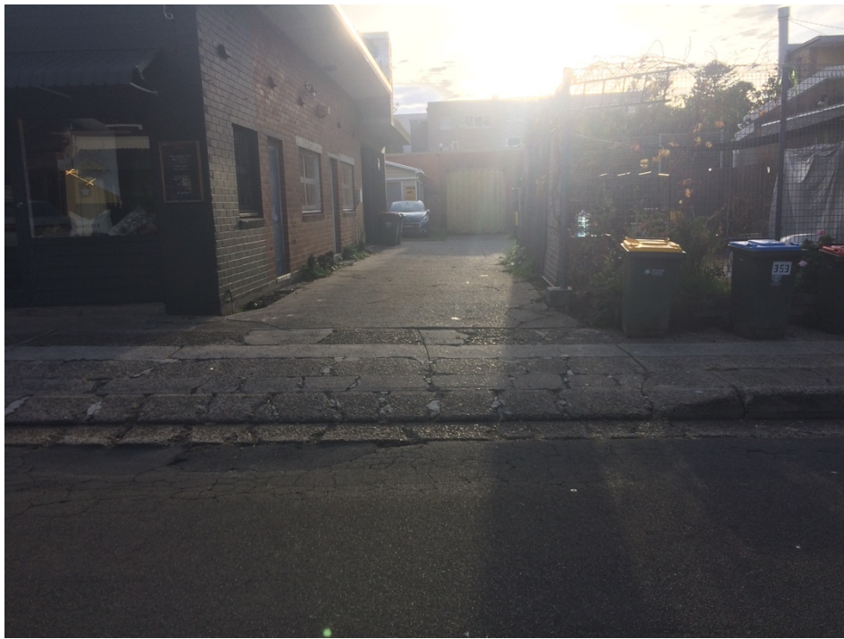
Photo 1 Driveway via Robertson Road, cracks on concrete pavement
