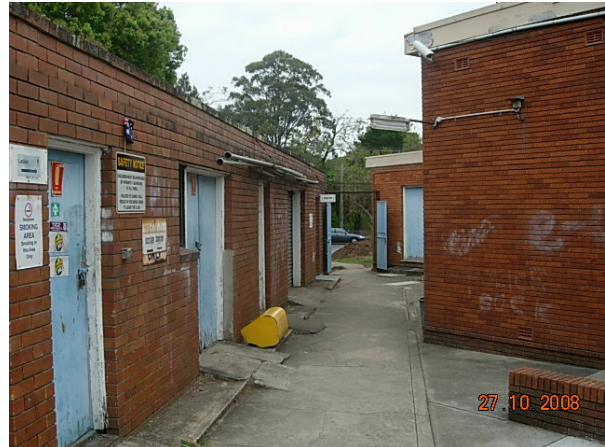
Photograph 4: Eastern elevation of existing club building (right) and men and women's change building (left) to be incorporated into the proposed extension.
