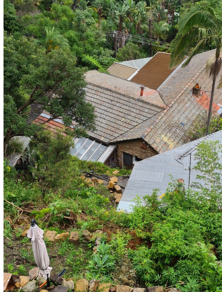
PHOTO 3 View from 6 Mitchell Road, showing slump/wall failure and flat sandstone bench with block debris at the rear of 17 Florida Road.
