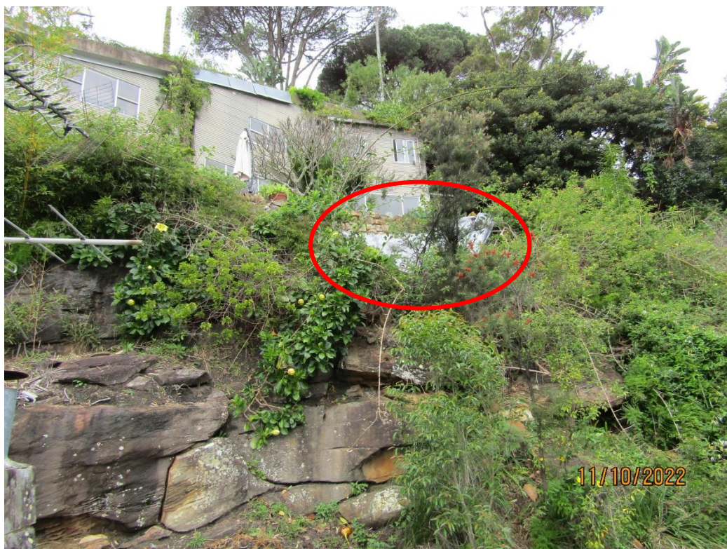
Photo 1 – failed portion of wall
