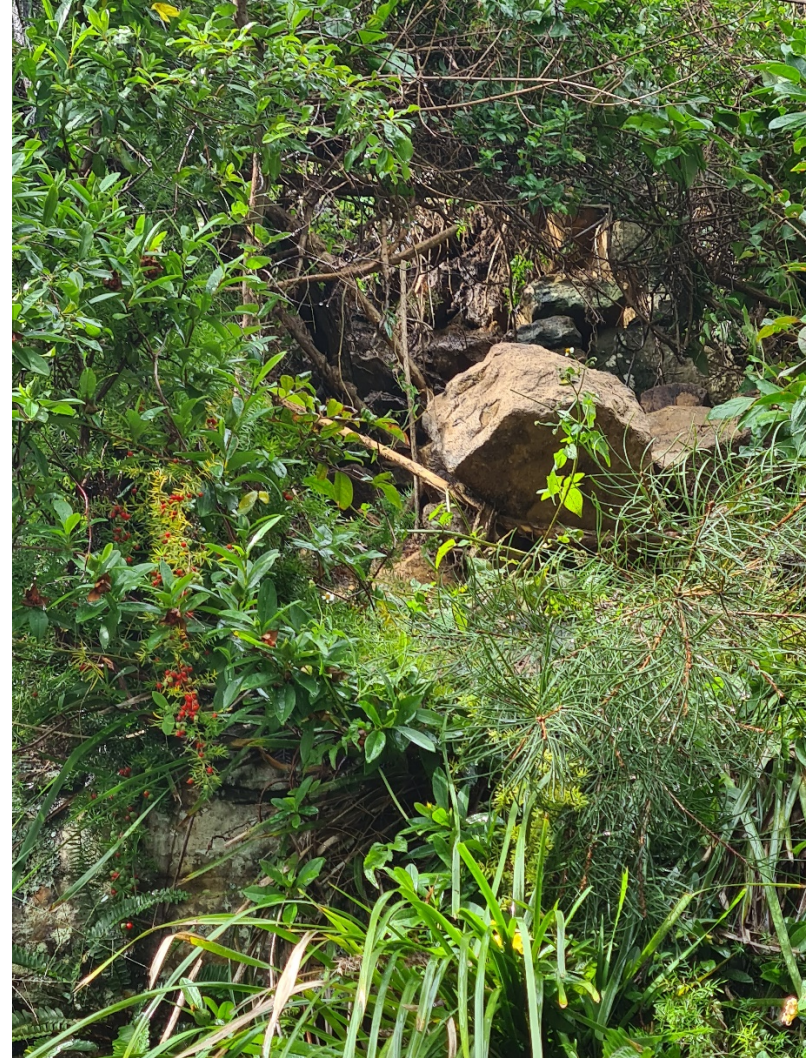
PHOTO 7 Close view of the unstable blocks above 17 Florida Road, the largest estimated as approximately 0.5 - 0.6 tonnes.
