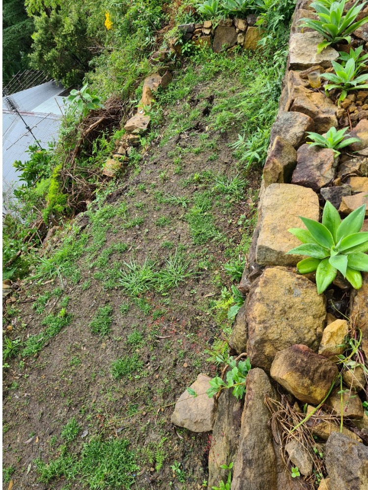
PHOTO 2 General view of slump area and failed lower retaining/landscape wall
