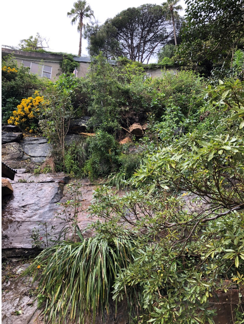
PHOTO 6 Three unstable blocks located approximately 10m above, and posing risk to the dwelling at 17 Florida Road.
