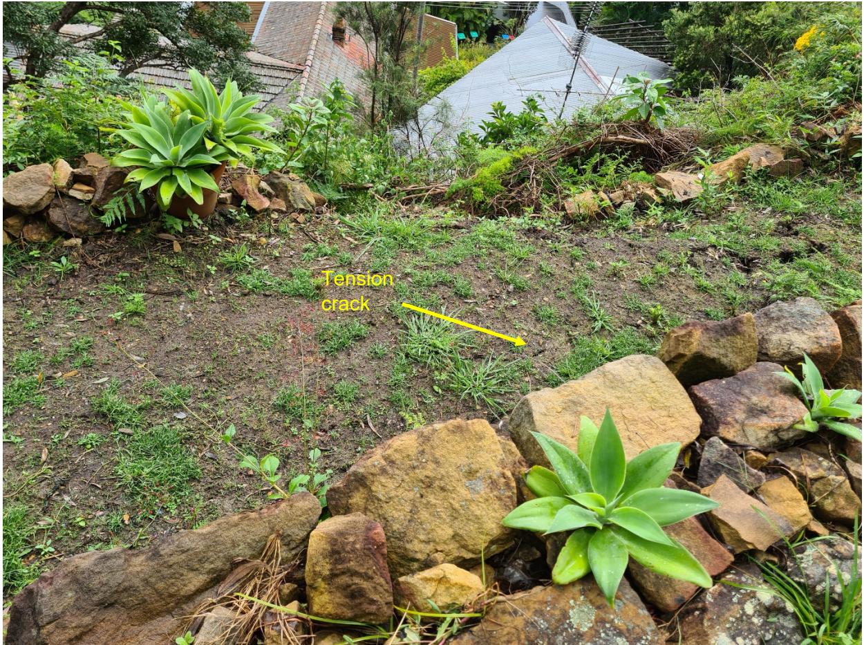
PHOTO 8 Small tension crack extending from slumped area, recommended to be filled with expanding foam filler.
