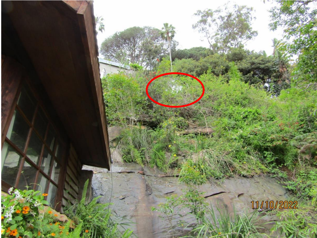
Photo 2 – failed portion of wall
