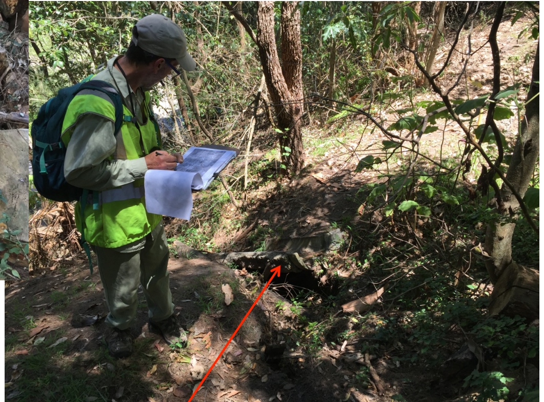
[Traverse T2] Half-round concrete batter drain eroded beneath by water from drainage line off No.83
