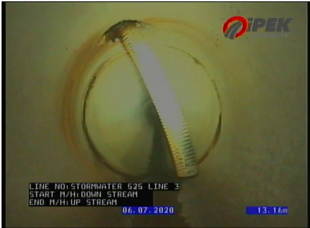
Photo: 6_6A 13.78m, Intruding connection, magnitude of intrusion: >75% , at 11 o'clock
