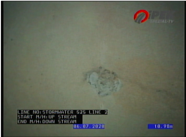
Photo: 2_8B 10.99m, Some coarse aggregate is visible , Obstruction: <5% , at 1 o'clock
