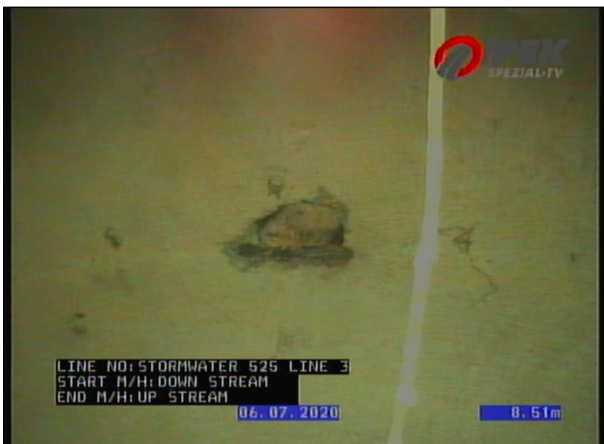
Photo: 3_6A 8.51m, Hole in wall , Obstruction: <5% , at 12 o'clock
