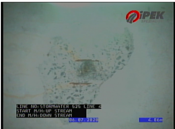
Photo: 4_2B 4.86m, Some coarse aggregate is visible , Obstruction: <5% , at 11 o'clock
