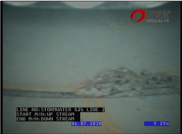
Photo: 2_7B 9.29m, Breaking, all pieces are present but some of them are visibly displaced from position, length of break 100 , from 12 to 12 o'clock
