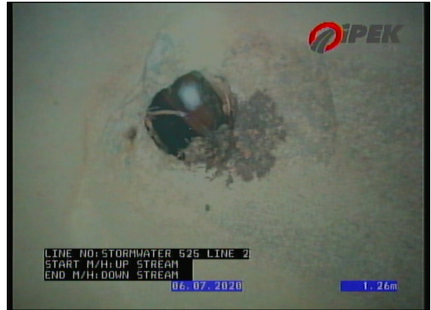
Photo: 2_2A 1.26m, Connection, good workmanship, connection appears to be open, height 50mm , at 2 o'clock
