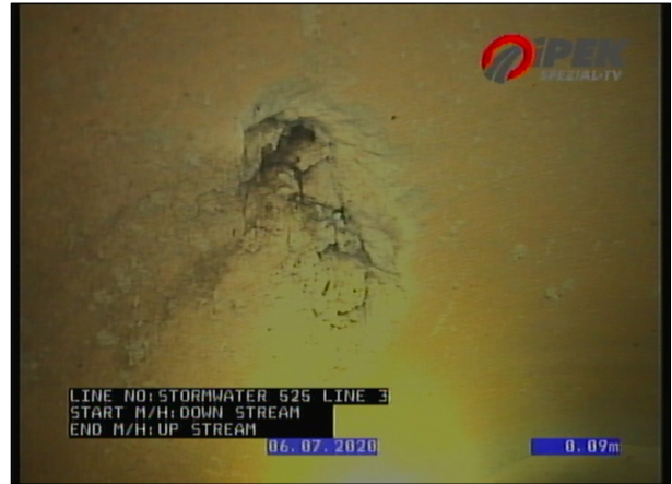
Photo: 6_2A 0.09m, Breaking, all pieces are present but some of them are visibly displaced from position, length of break 100 , at 10 o'clock
