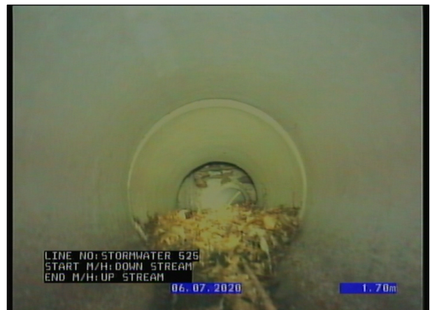
Photo: 4_3A 2.92m, Inspection (survey) abandoned, Build up of leaves from pit
