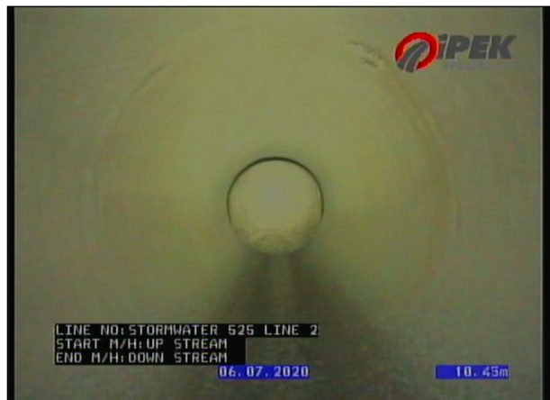
Photo: 2_8A 10.99m, Some coarse aggregate is visible , Obstruction: <5% , at 1 o'clock
