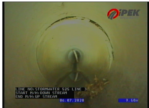
Photo: 6_5A 10.41m, Joint displaced radially, radial displacement 11-20mm , at 1 o'clock
