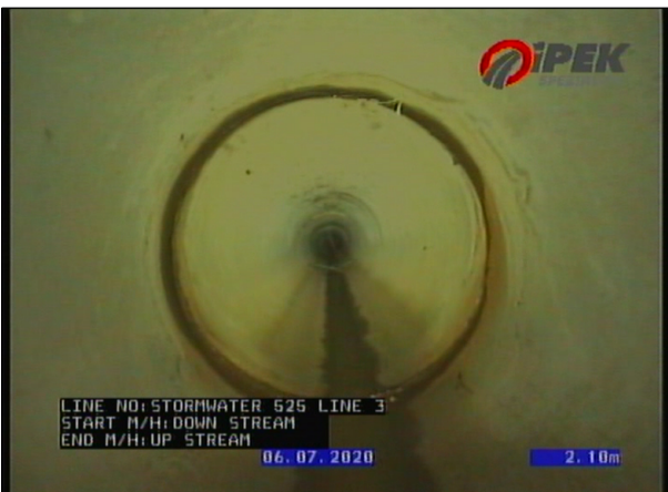
Photo: 6_3A 2.88m, Infiltration, sweating, at joint , from 12 to 12 o'clock
