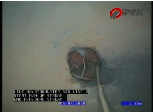
Photo: 2_4B 3.25m, Connection, good workmanship, connection appears to be open, height 50mm , at 1 o'clock
