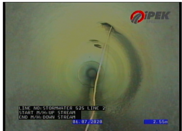
Photo: 2_4A 3.25m, Connection, good workmanship, connection appears to be open, height 50mm , at 1 o'clock
