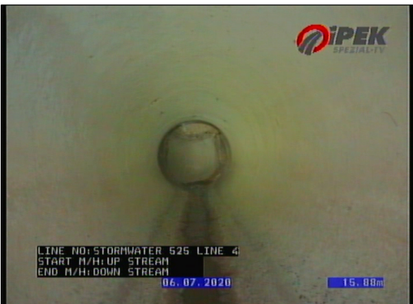
Photo: 4_4A 15.88m, Inspection (survey) abandoned, Buildup of leaves
