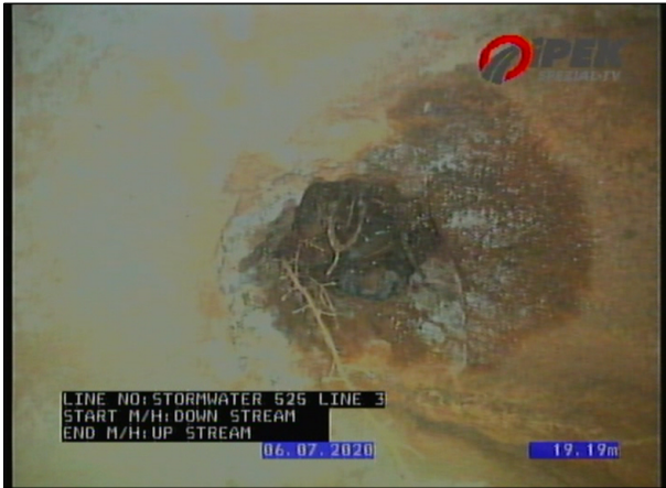
Photo: 6_9B 19.19m, Infiltration, sweating , at 1 o'clock
