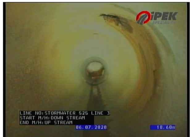
Photo: 6_9A 19.19m, Infiltration, sweating , at 1 o'clock
