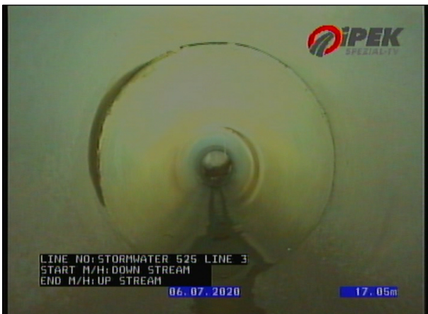
Photo: 6_8A 17.77m, Infiltration, sweating, at joint , at 10 o'clock
