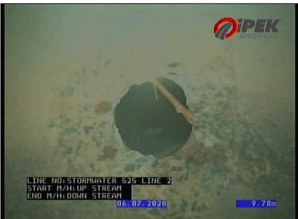
Photo: 2_9B 9.78m, Connection, poor workmanship, connection appears to be open , height 50mm
