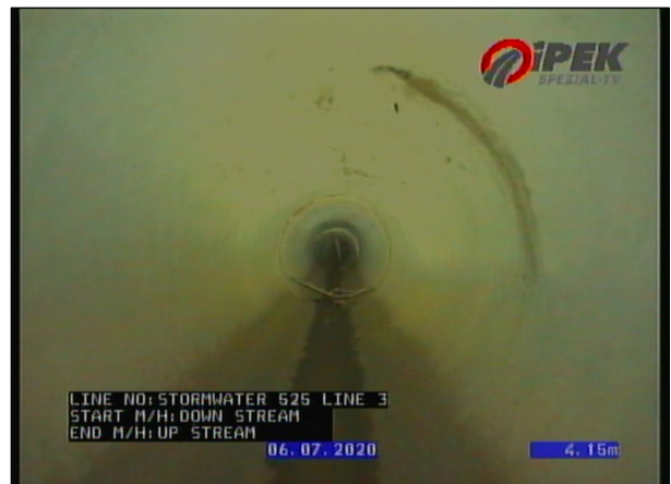
Photo: 6_4A 4.72m, Infiltration, sweating , at 1 o'clock
