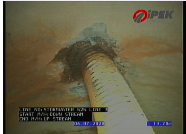
Photo: 6_6B 13.78m, Intruding connection, magnitude of intrusion: >75% , at 11 o'clock
