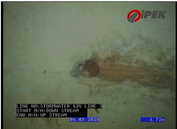
Photo: 6_4B 4.72m, Infiltration, sweating , at 1 o'clock
