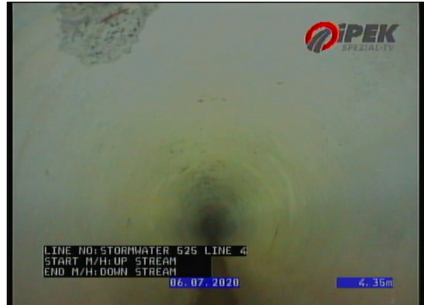
Photo: 4_2A 4.86m, Some coarse aggregate is visible , Obstruction: <5% , at 11 o'clock
