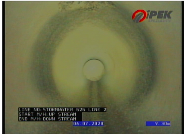
Photo: 2_9A 9.78m, Connection, poor workmanship, connection appears to be open , height 50mm
