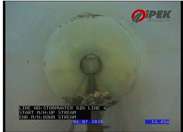
Photo: 4_3A 15.42m, Joint displaced radially, radial displacement 5-10mm , at 1 o'clock
