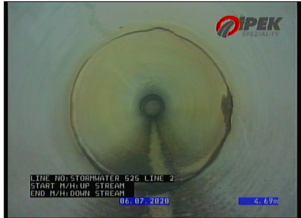
Photo: 2_7A 5.53m, Infiltration, sweating, at joint , from 3 to 7 o'clock
