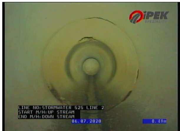
Photo: 2_7A 9.29m, Breaking, all pieces are present but some of them are visibly displaced from position, length of break 100 , from 12 to 12 o'clock
