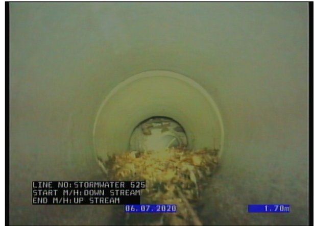
Photo: 4_2A 2.64m, Joint displaced radially, radial displacement 5-10mm , at 12 o'clock
