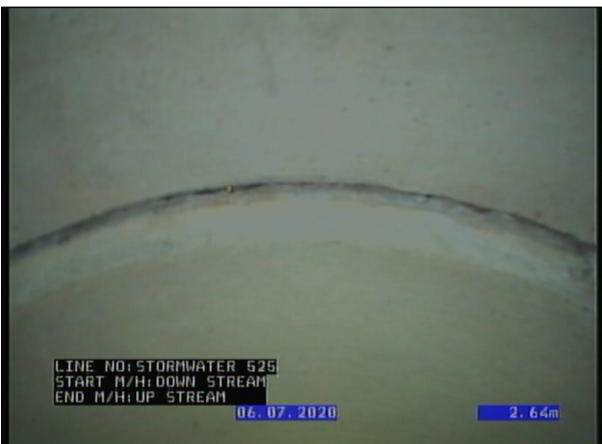
Photo: 4_2B 2.64m, Joint displaced radially, radial displacement 5-10mm , at 12 o'clock
