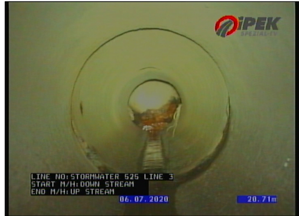
Photo: 6_10A 21.48m, Hard or compacted material in the invert, at joint, Obstruction: <5% , from 7 to 8 o'clock
