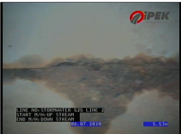
Photo: 2_7B 5.53m, Infiltration, sweating, at joint , from 3 to 7 o'clock
