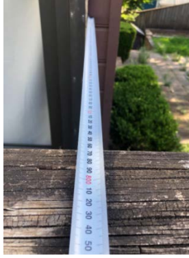
Picture taken of measurement of proposed fire egress path less than 1m.
