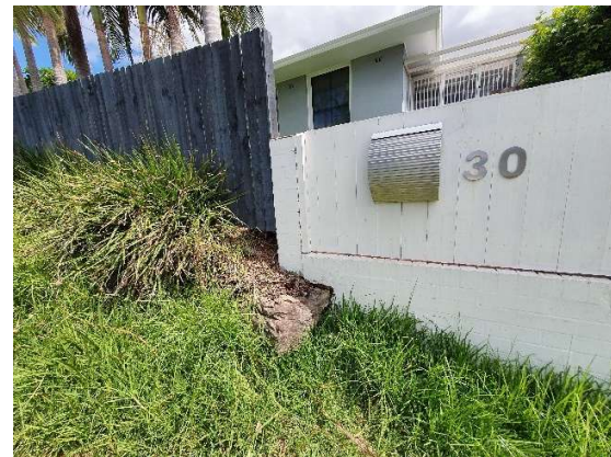
Photograph-16: Bedrock outcrop at the base of the boundary wall. View looking west.
