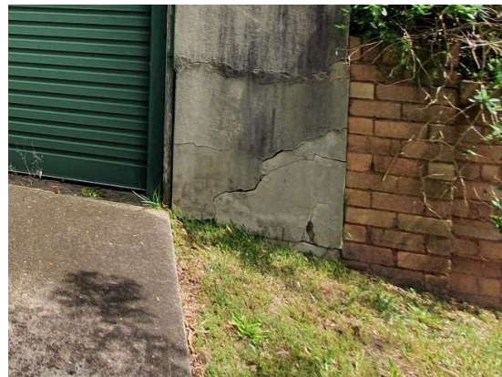
Photograph-9: Rendered brick garage defect. View looking west.
