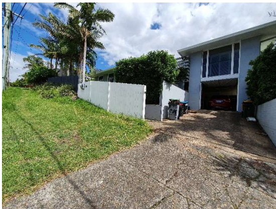
Photograph-15: Cracks within the concrete driveway. View looking west.
