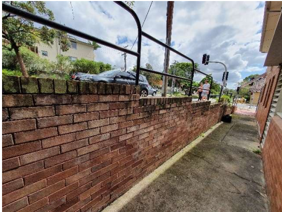
Photograph-13: Brick retaining wall to the west of concrete pathway. View looking north.
