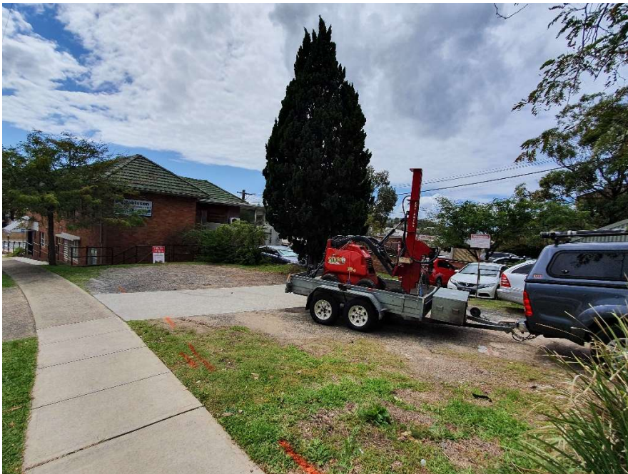
Photograph-3: Rear of the site from the south west corner of the site. View looking north.
