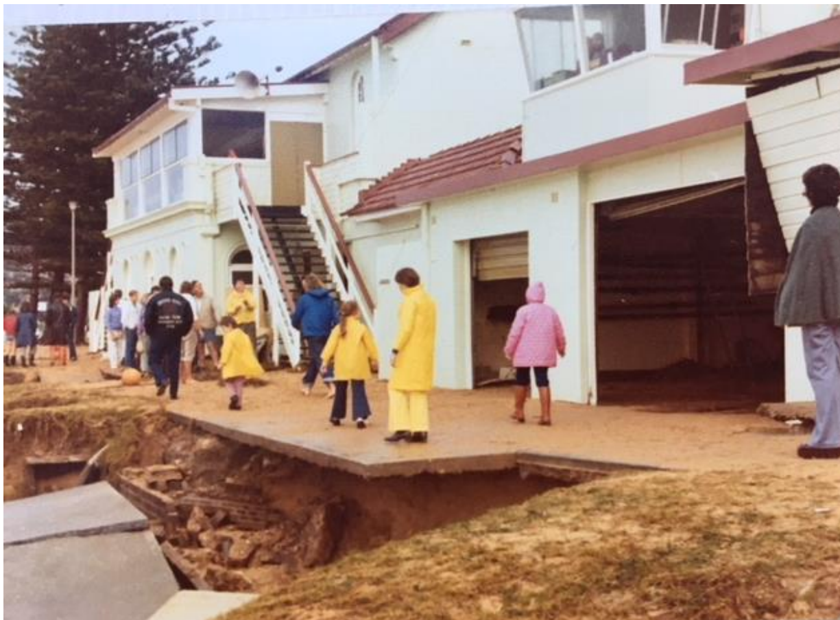
Figure 4: Damage to Newport SLSC from coastal storm in May 1974
