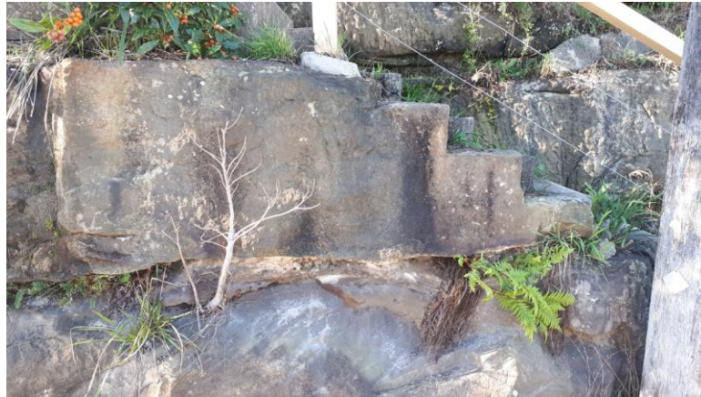
Photo 4: Stairway founded on undercut bed of sandstone
