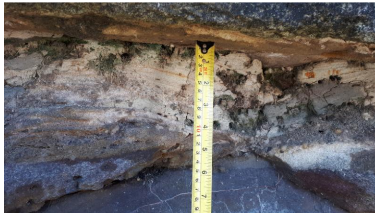
Photo 5: Clay seam below the undercut rock
