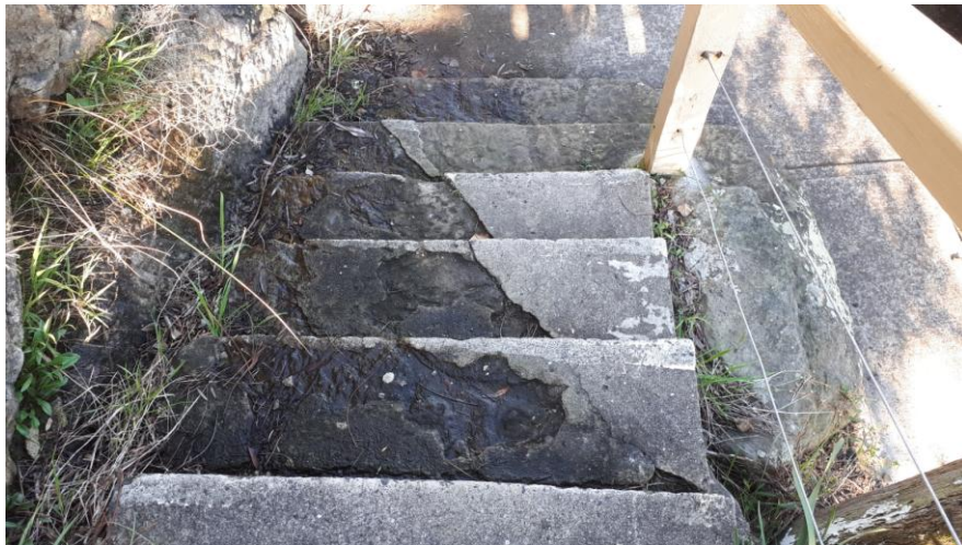
Photo 2: Uneven and slippery rock surface over the bottom steps
