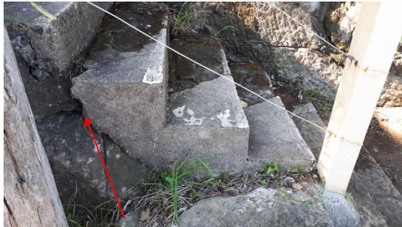
Photo 3: Crack between concrete steps
