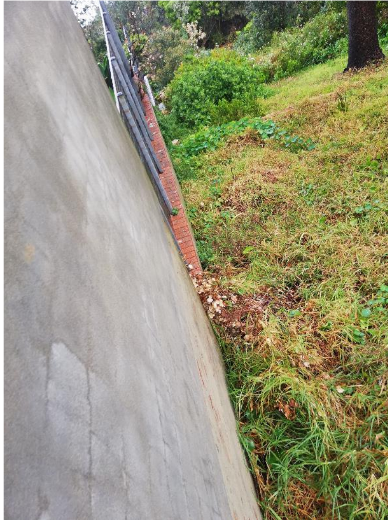
Image 4. View of Retaining Wall Render From Neighbouring Property
