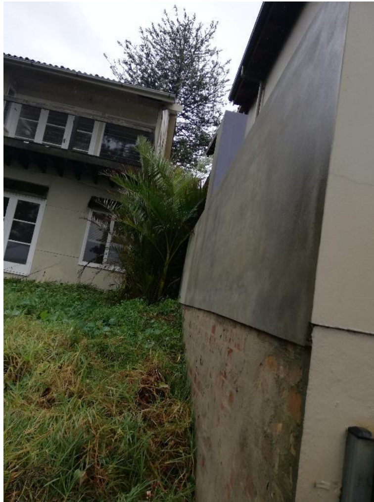
Image 5. View of Retaining Wall Render From Neighbouring Property
