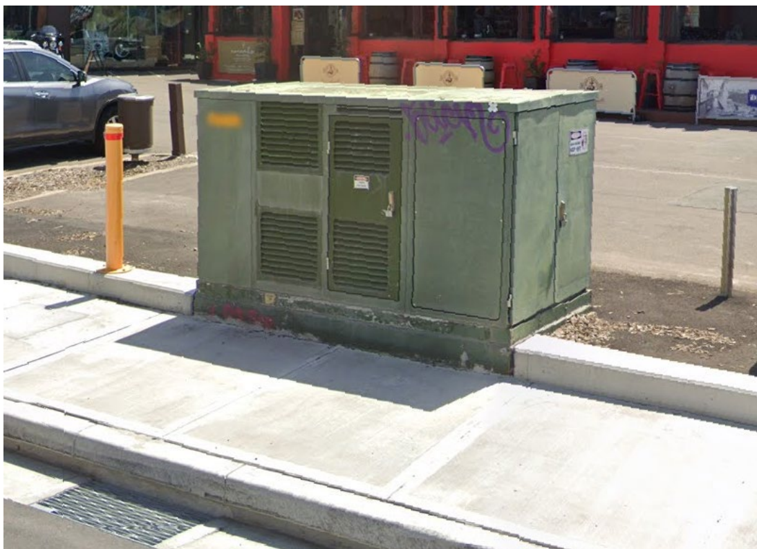
Figure 1 Typical existing Ausgrid transformer kiosk, as the basis for the JUMP charging stations
