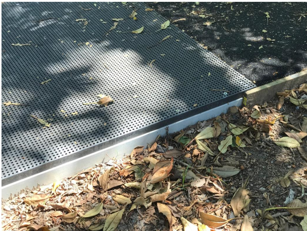
Plate 2 – Typical elevated FRP walkway interface with asphalt path (St. Leonards Park, North Sydney)
