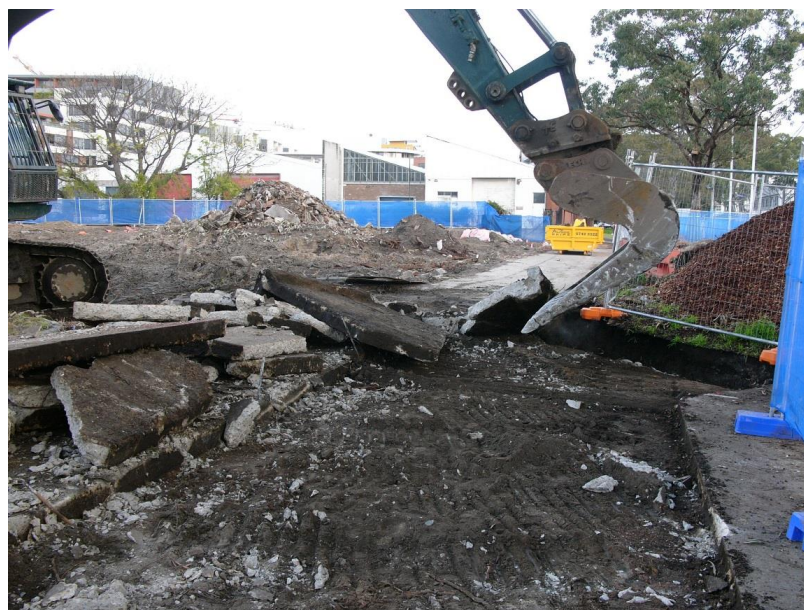
Figure 2 – Showing method for removal of concrete pavement, by carefully lifting sections and folding over the remaining paved surface.
