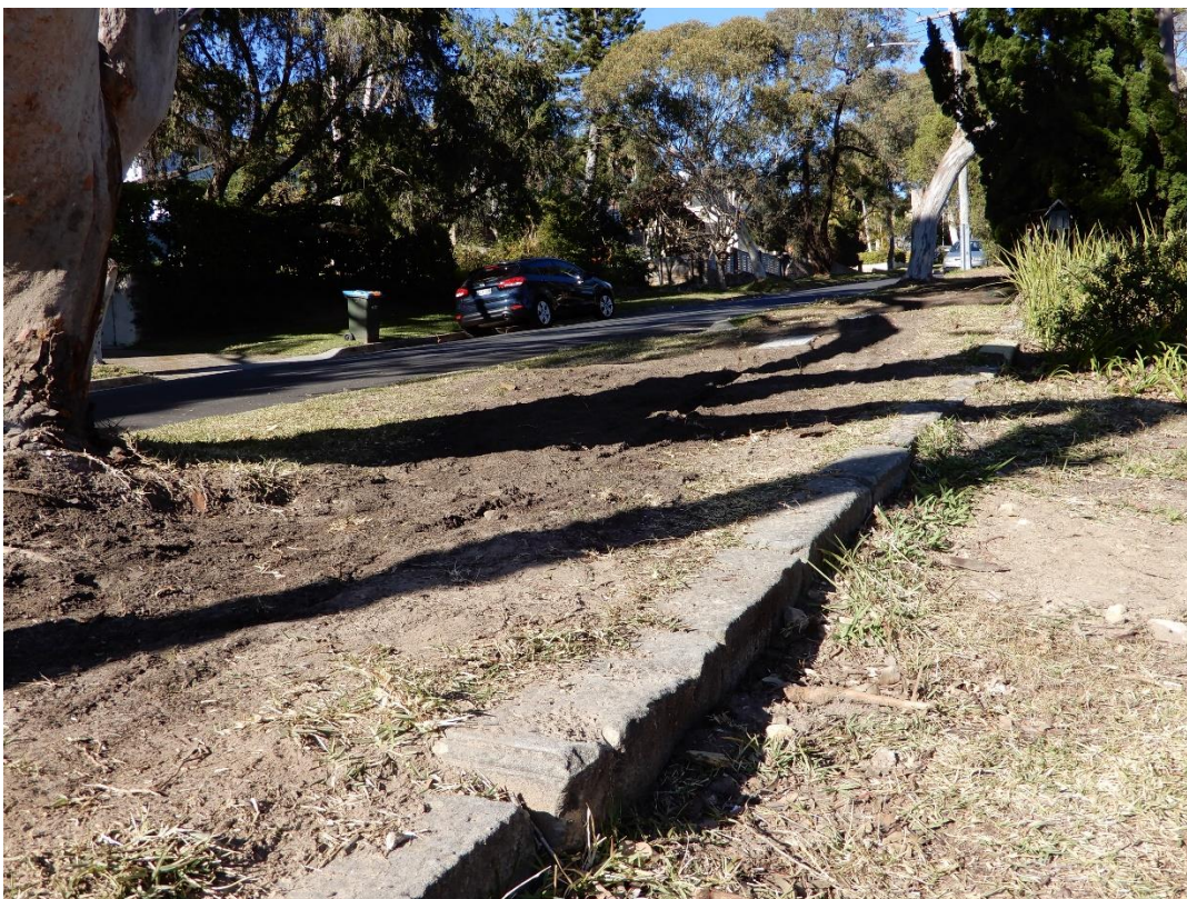
Photograph 6: Tree # 3 – Illustrating the level drop into the site in TPZ/SRZ of the tree.
