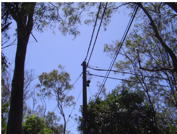
Electrical supply connection point
