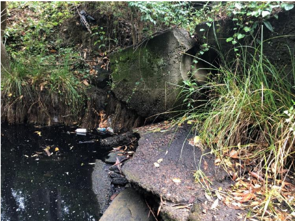
Plate 1. Damaged headwall to be repaired
