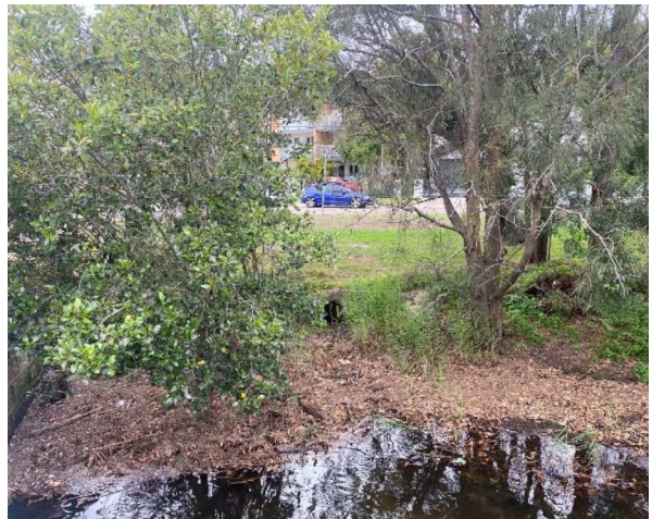
Figure 44: View north towards approximate works area showing drainage culvert and regrowth vegetation along Manly Creek
