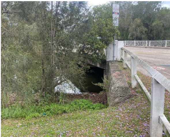
Figure 43: View south-west showing concrete footings of existing pedestrian footbridge along Pittwater Road and approximate works area
