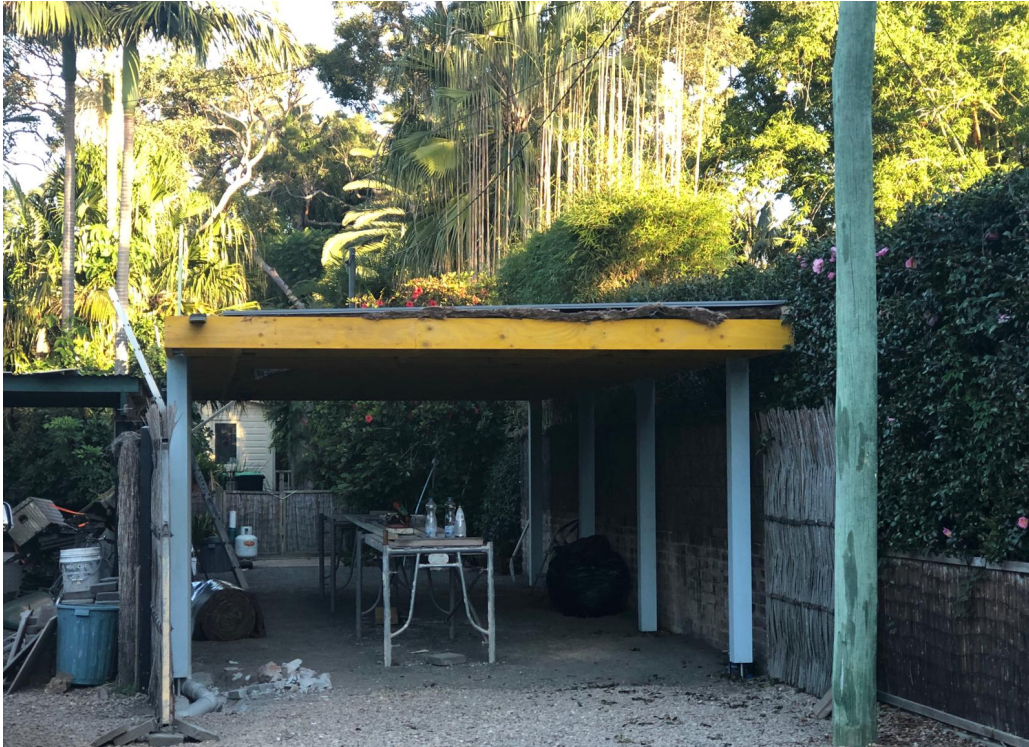
Figure 1: View of unauthorised carport from Joseph Street, facing south-east
