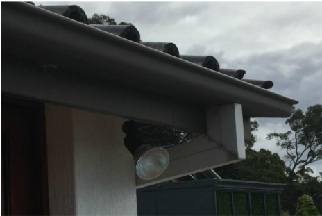
MONUMENT FACIA, GUTTER & DOWNPIPES
