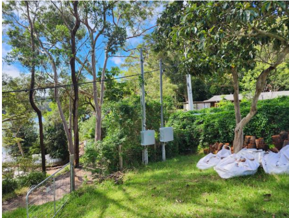
Existing electrical supply
