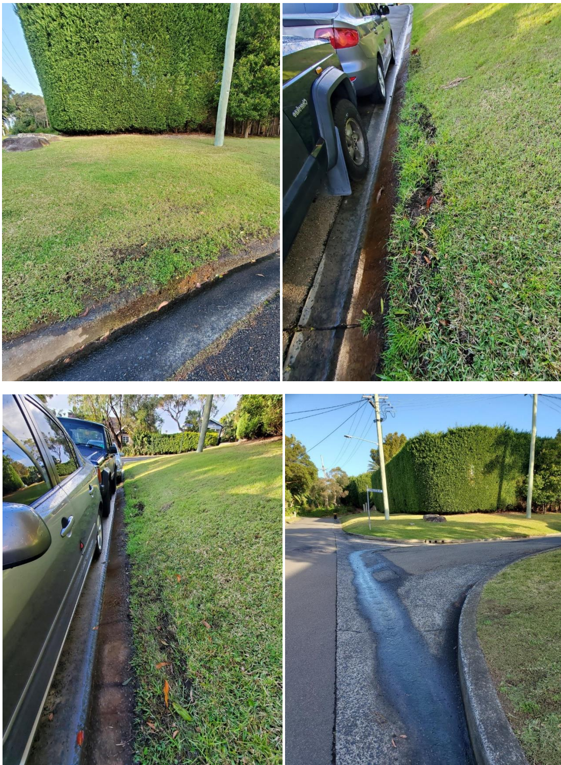
Figure 5: Continual seepage/runoff from 106 Bynya Road along boundary with Ralston Road and intersection of Ralston Road and Bynya Road showing saturation of verge and chronic nature of this issue
