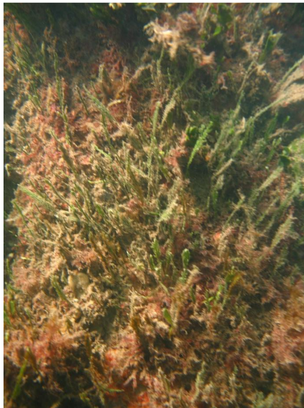
Figure 15. The invasive and noxious algae Caulerpa taxifolia and turfing algae colonising a pile supporting the jetty.
