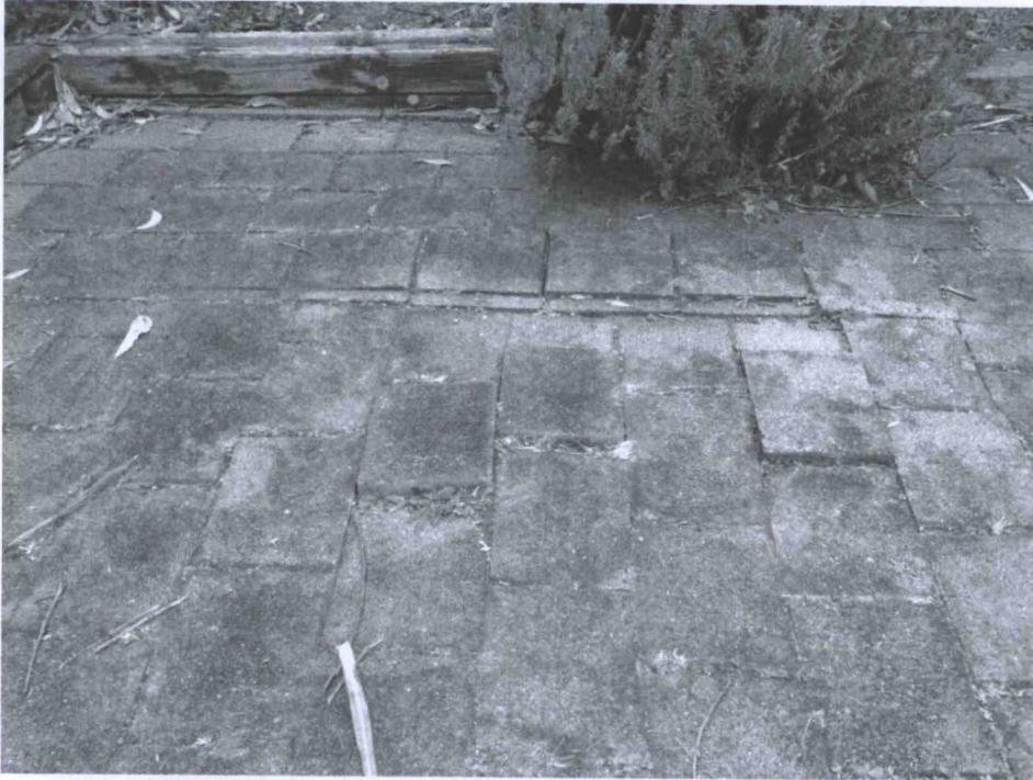
Pictures showing root damage caused by tree.
