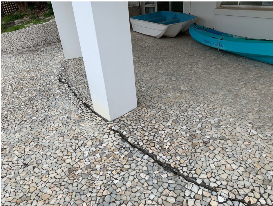
Photo 2 Evidence of ground settlement at rear terrace of the Site.
