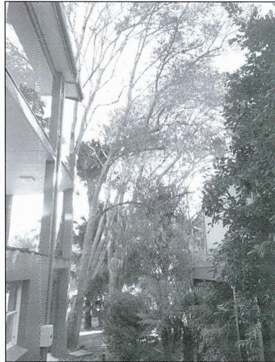
Figure 16: Trees leaning toward neighbouring property.
