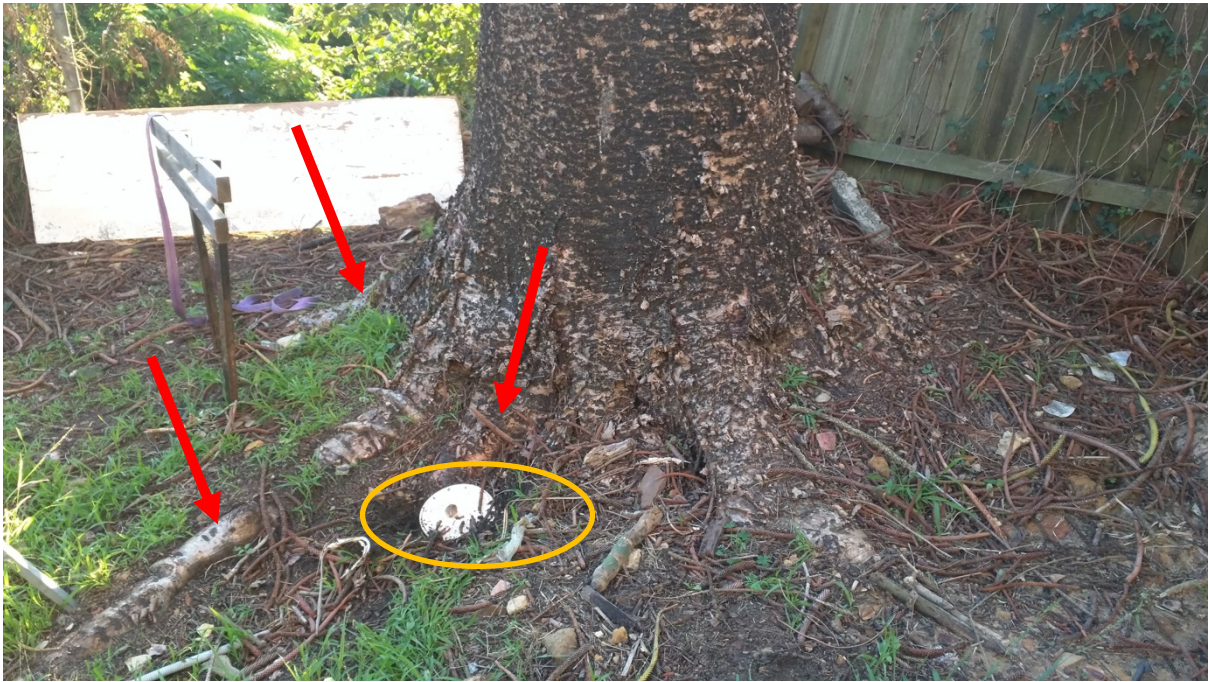
Photo 3: Base of tree showing lateral roots orientating towards pool (red arrow) and a sewer inspection cap (yellow).
