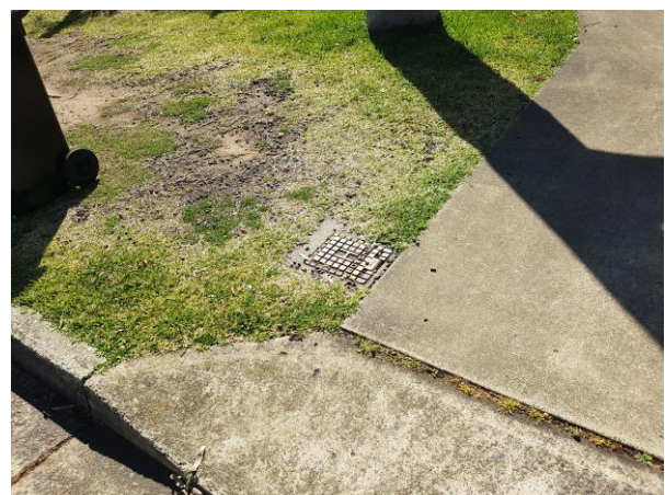
Reticulated water hydrant in pathway
