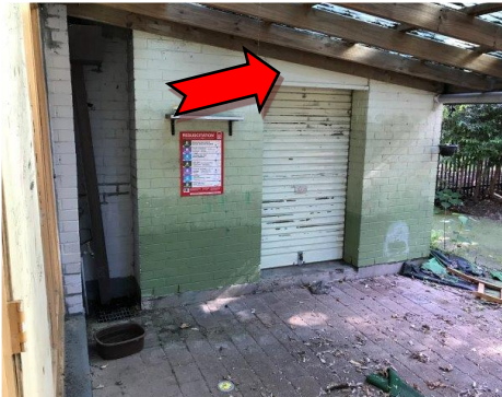
3. Exterior, adjacent north entrance, above roller door – asbestos-containing fibre cement sheet infill panel.
