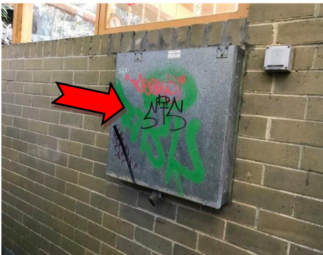
5. Exterior, south-west corner of building, inaccessible electrical box – asbestos-containing bituminous backing board assumed to be present within.
