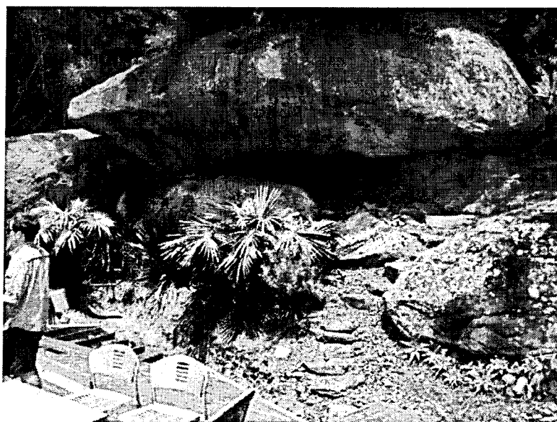
Photo: 3 – Large irregular shaped boulder within neighbouring property, sitting atop two small boulders and of very poor shape and position for long term stability.
