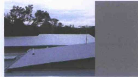
MR: Colorbond "Windspray" steel roof sheeting
