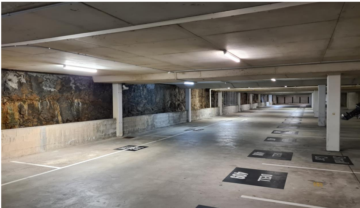
Photo 14 - BEDROCK Unit Observed in B2
