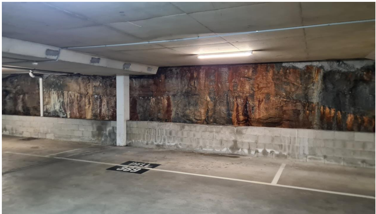
Photo 12 - BEDROCK Unit Observed in B2
