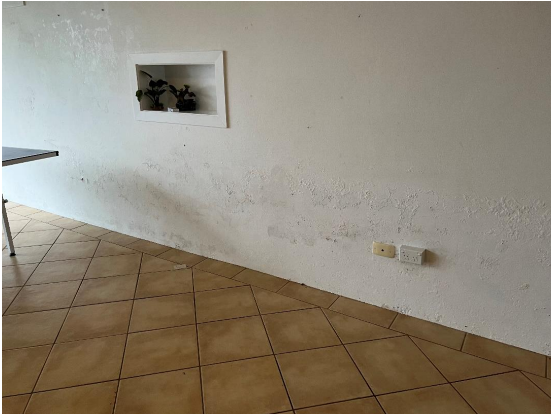
Photo of water damage to the existing lower ground room fronting Marine Parade, 02.02.22, Squillace Architects
