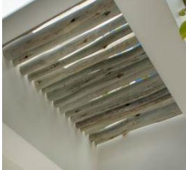
TM01 LATHS ABOVE PERGOLA TIMBER: WEATHERED
