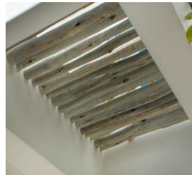
TM01 LATHS ABOVE PERGOLA TIMBER: WEATHERED
