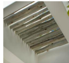
TM01 LATHS ABOVE PERGOLA TIMBER: WEATHERED
