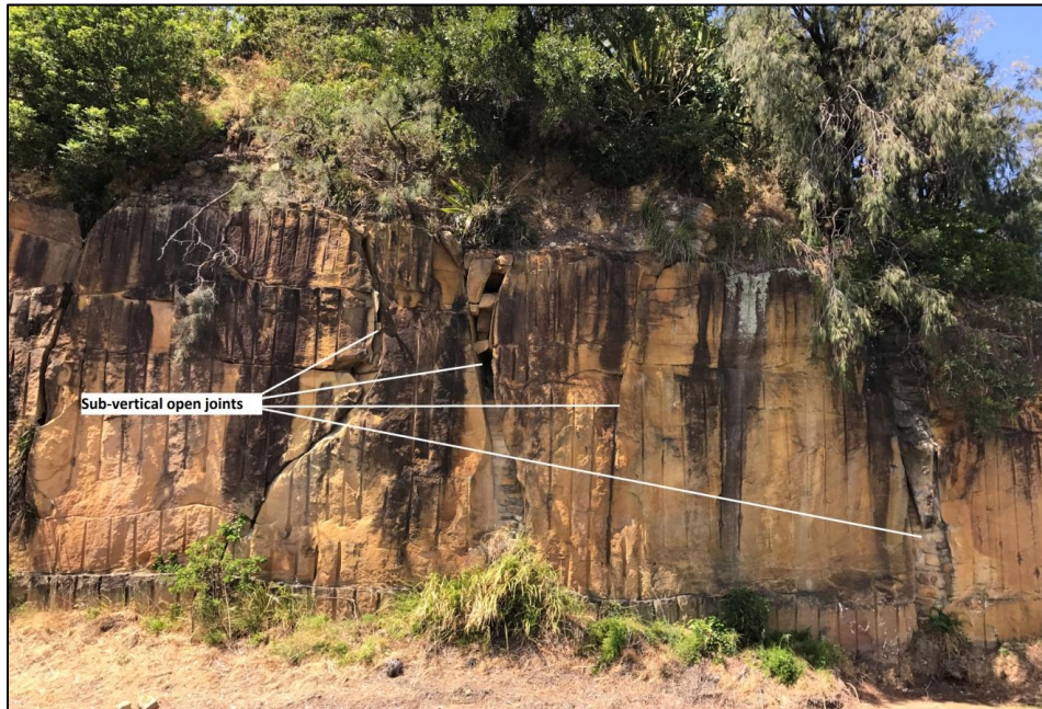
Photograph 6: View of defects within exposure to the west of the site
