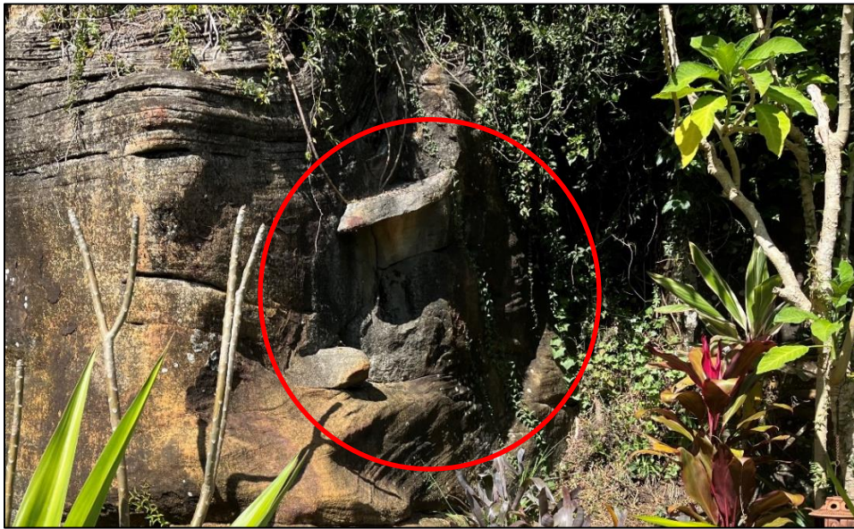
Photograph 4: View of a previous wedge failure (circled red) within the cliff line to the rear of the site house.
