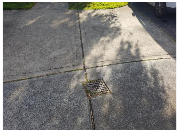
Reticulated water hydrant in pathway
