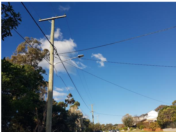
Above ground electrical supply
