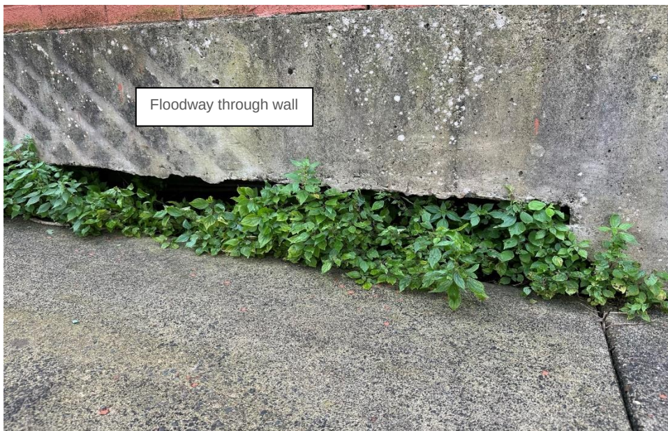
Photo 2: Southern boundary where flood flows enter the site
