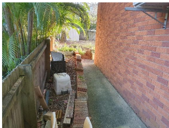
Photograph-6: Tilted brick retaining wall along the south boundary. View looking west.
