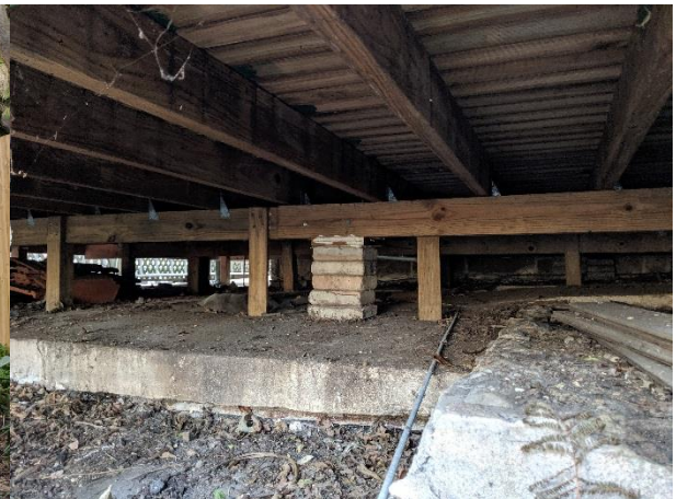
Figure 7. Cavity under the existing deck.
