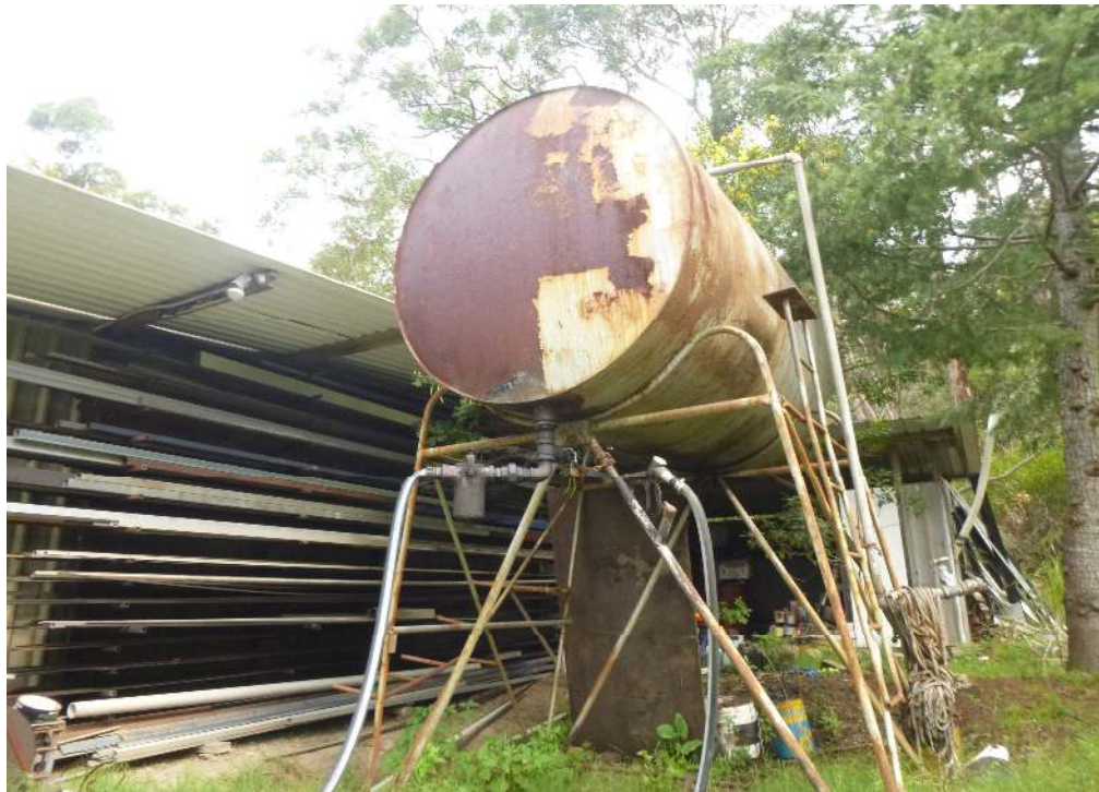
Photograph 11 - Above Ground Storage Tank
