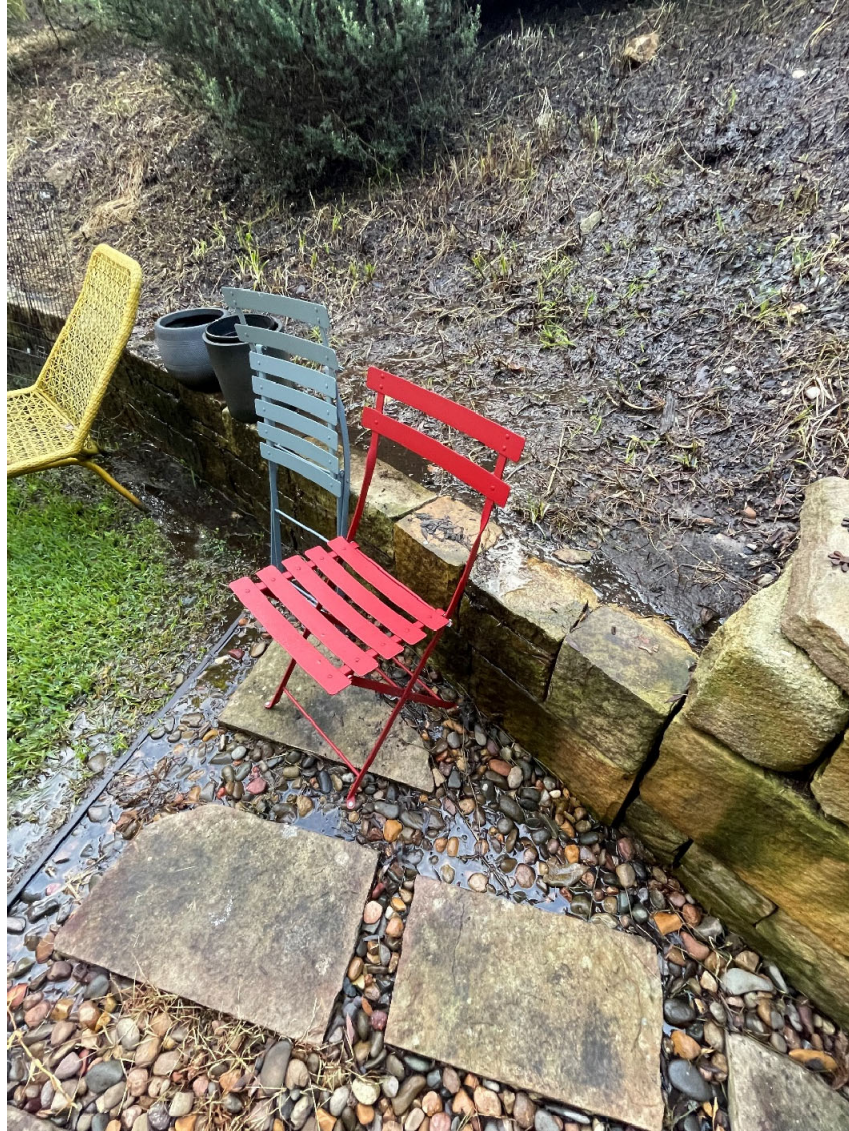
Image 4. Showing onsite drainage issues and water inundation at base of existing wall.
