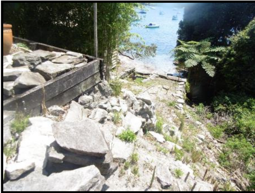
Existing planting and failed retaining walls in area of the proposed inclinator
