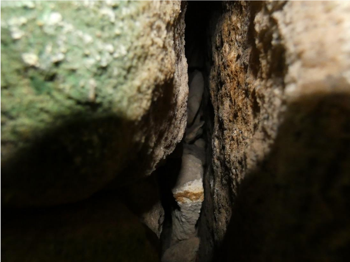
Photo 9: Example of a cavity in the sandstone retaining wall.
