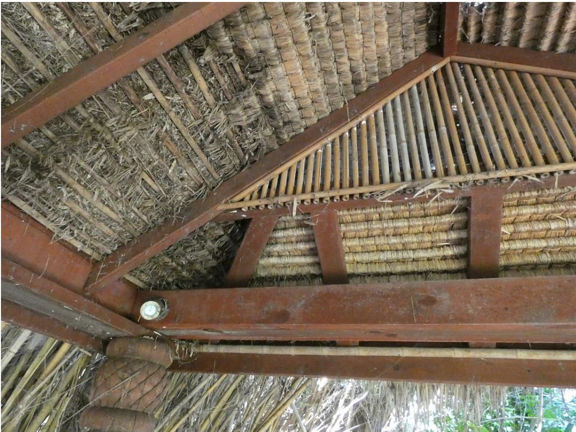
Photo 6: The underside of the gazebo roof was assessed as potential roosting habitat for microbats.
