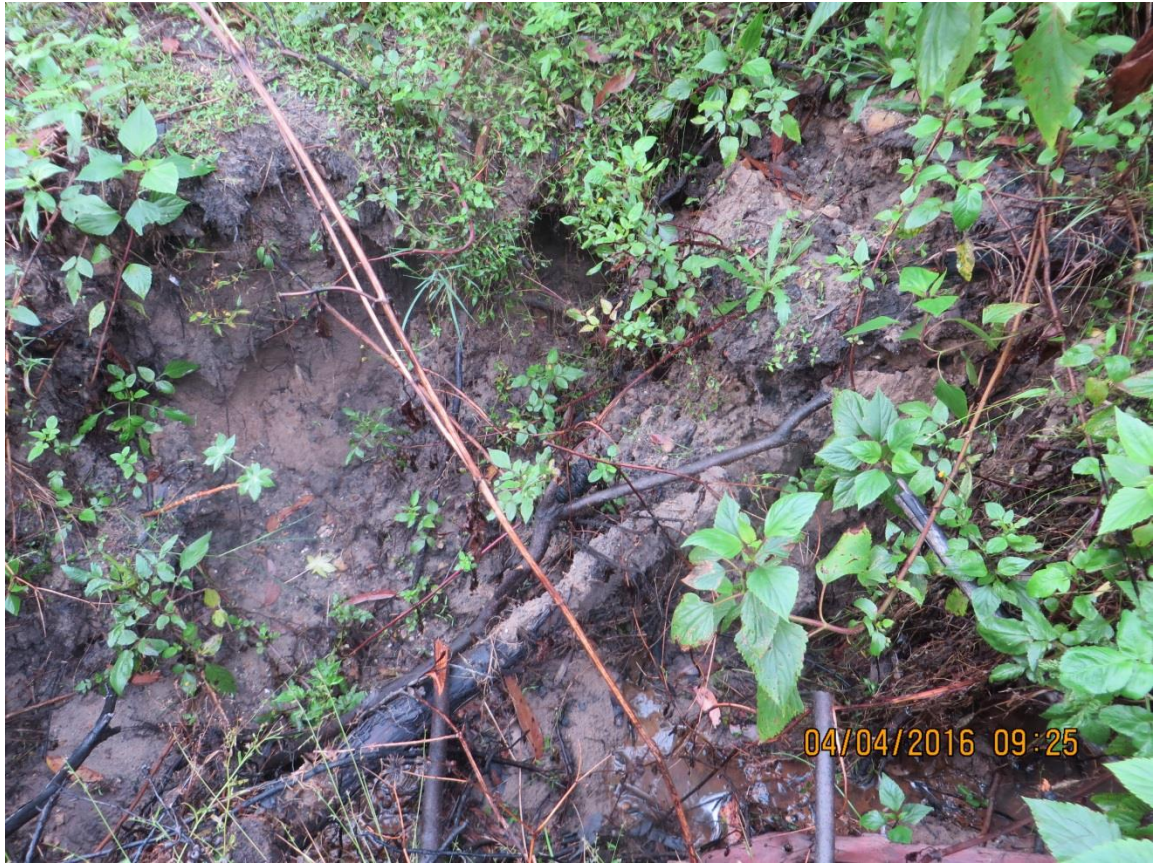
Figure 6. Site 4. The heavy rainfall has cause local instability of the banks (339315 6264907).
