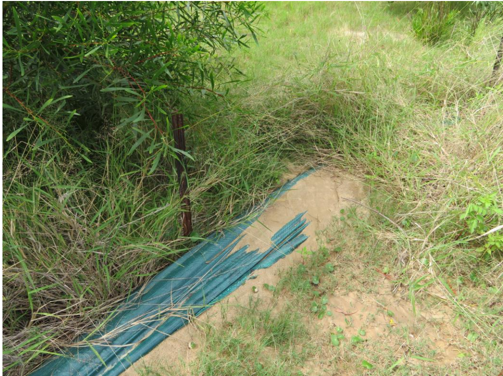
Figure 2.14. The silt fence parallel to the northern border in March 2017. The native couch grass sward is providing an effective sediment trap. There is minimal 'escape' of sand off the lot and moving north.
