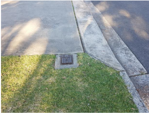
Reticulated water supply along Beatty Street
