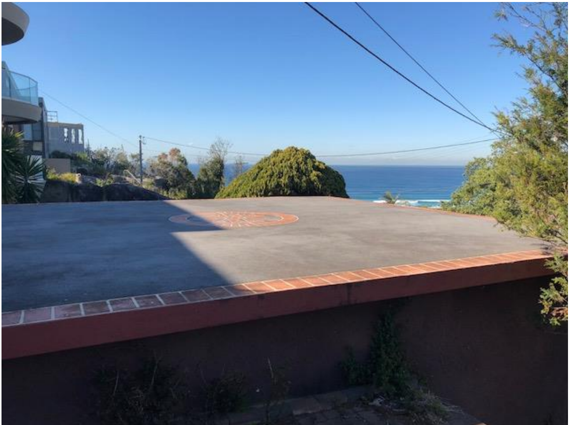
Figure 6. Existing garage roof / patio accessed from front garden area
