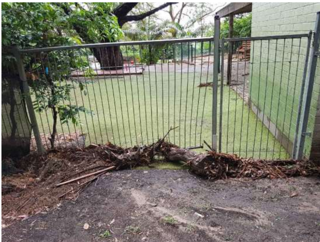
Figure 4: Damaged caused to fencing at the preschool from flooding – March 2018
