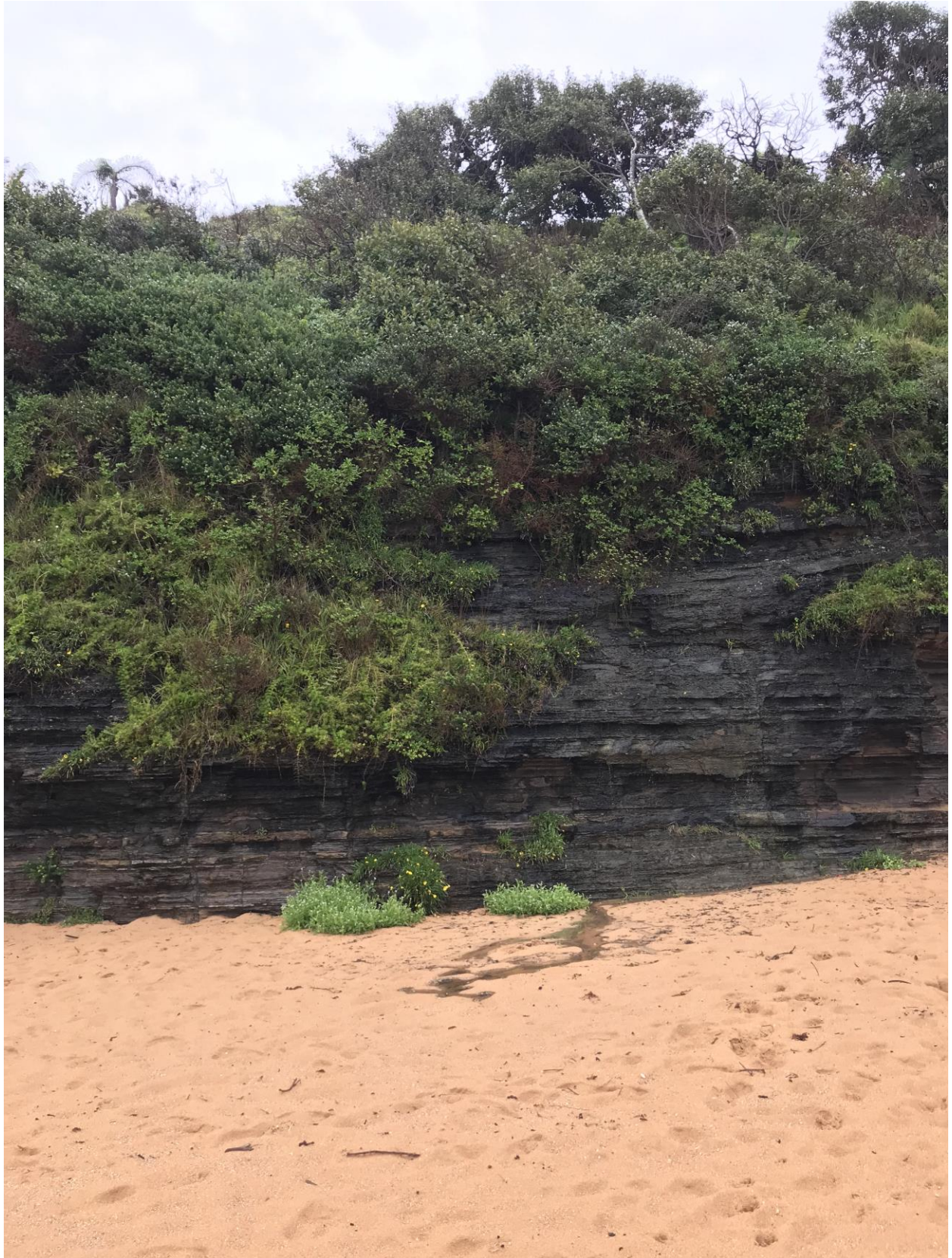
Figure 4: Close view of cliff face SE of subject property on 25 February 2022, facing NW to NNW
