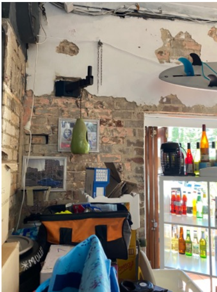
Figure 26.0, Render partially removed from brickwork, AW 2020
