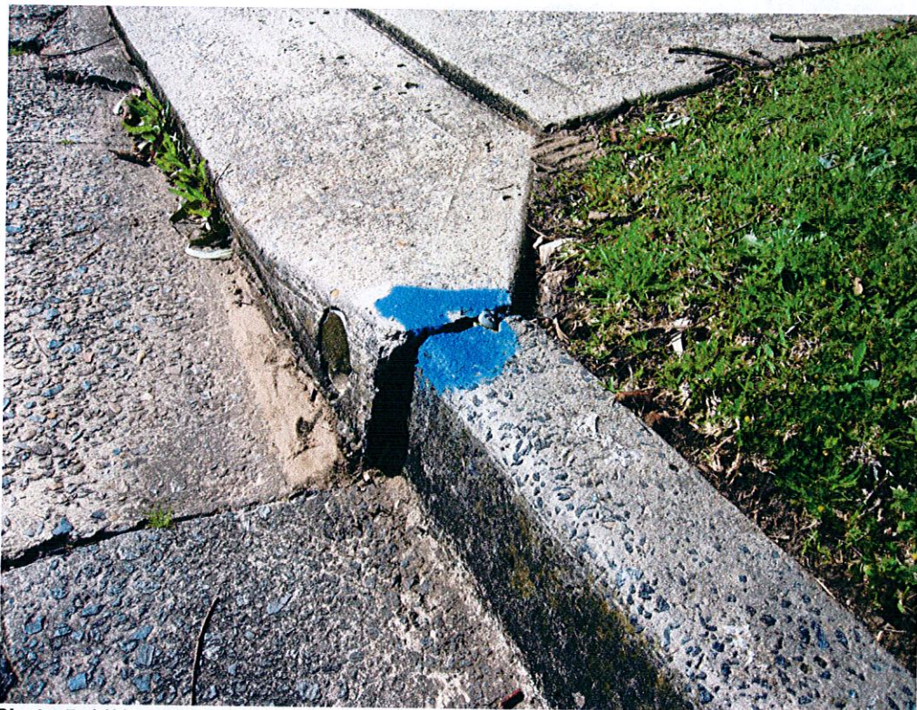
Photo 5: Lifting and buckling of the concrete kerb and cracks in the gutter to 6 Gordon street.
