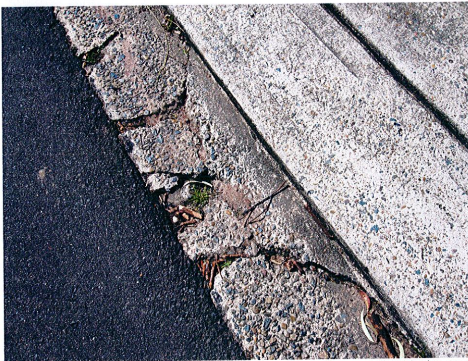
Photo 4: Viewing cracks and decrepit concrete gutter to the council vehicular crossover to 6 Gordon Street.
