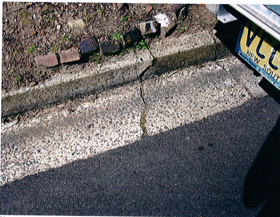
Photo 6: Lifting and cracking of the concrete kerb and lifting of brick edging to 6 Gordon street.
